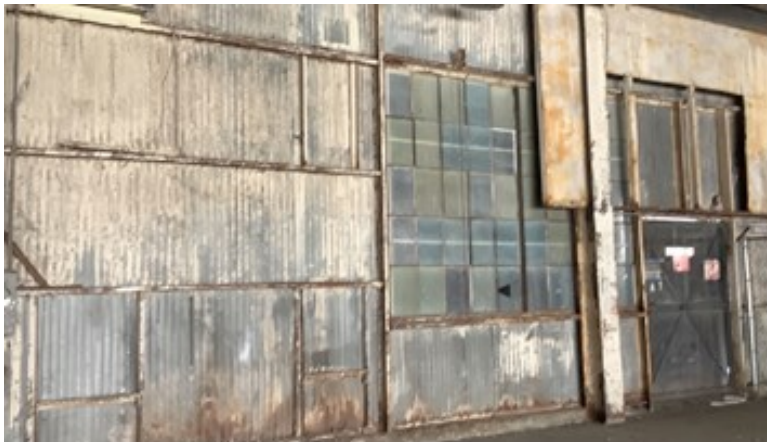
Photo 1 Dilapidated Structures on OTC (Exterior)
